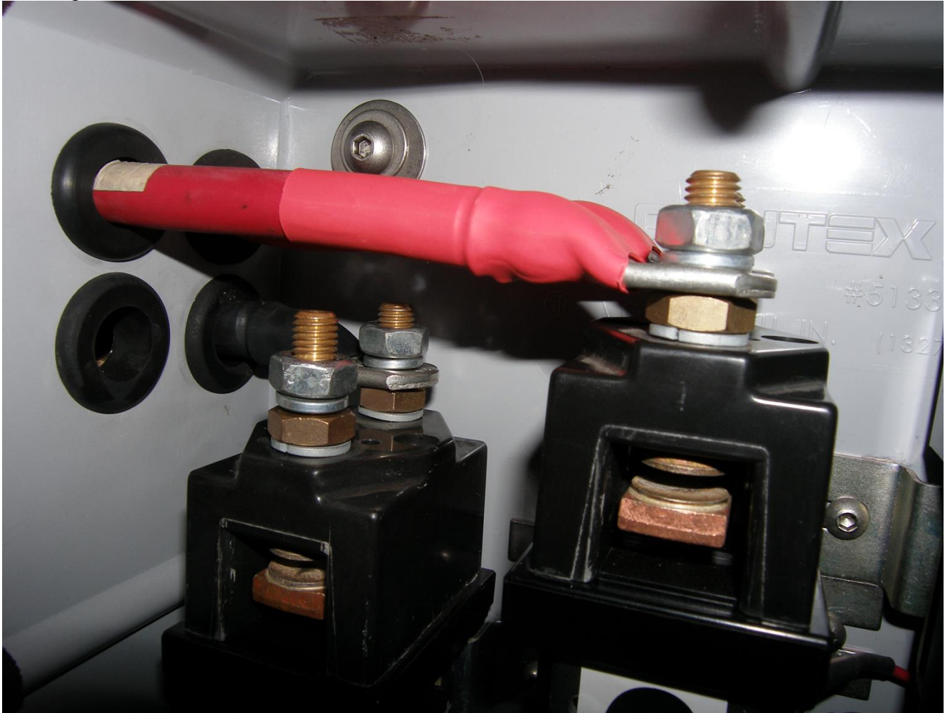
Figure 8 – 10 Cables rule. Note the rubber grommets fixed in the holes.
